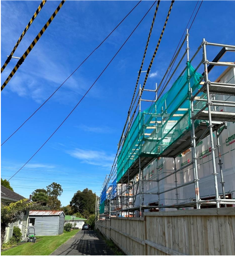
Figure 3: Non-compliant building and scaffold near 400V lines. Unauthorised third-party insulation was applied by an unknown person.
