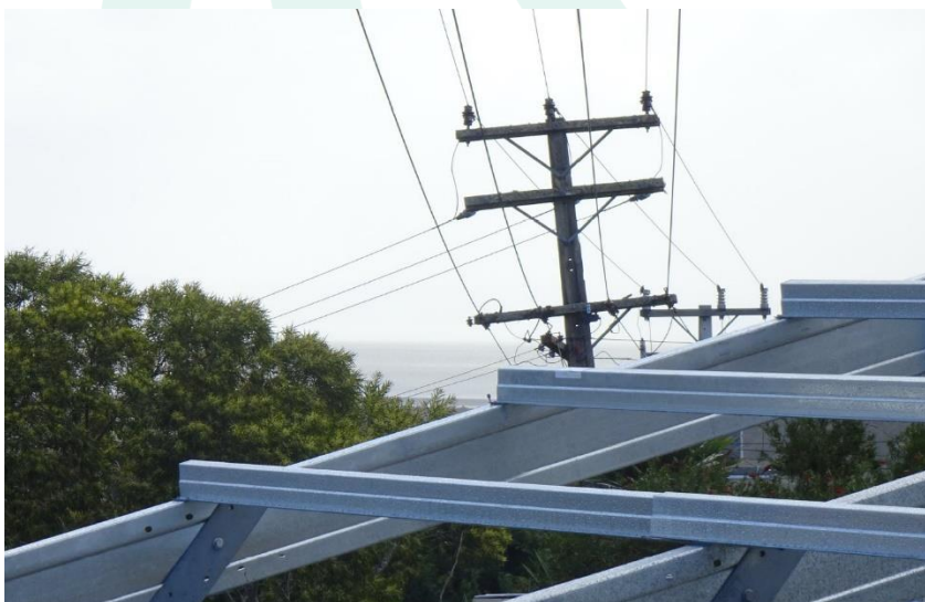
Figure 2: Non-compliant rural building below 400v and 11 kV lines.
