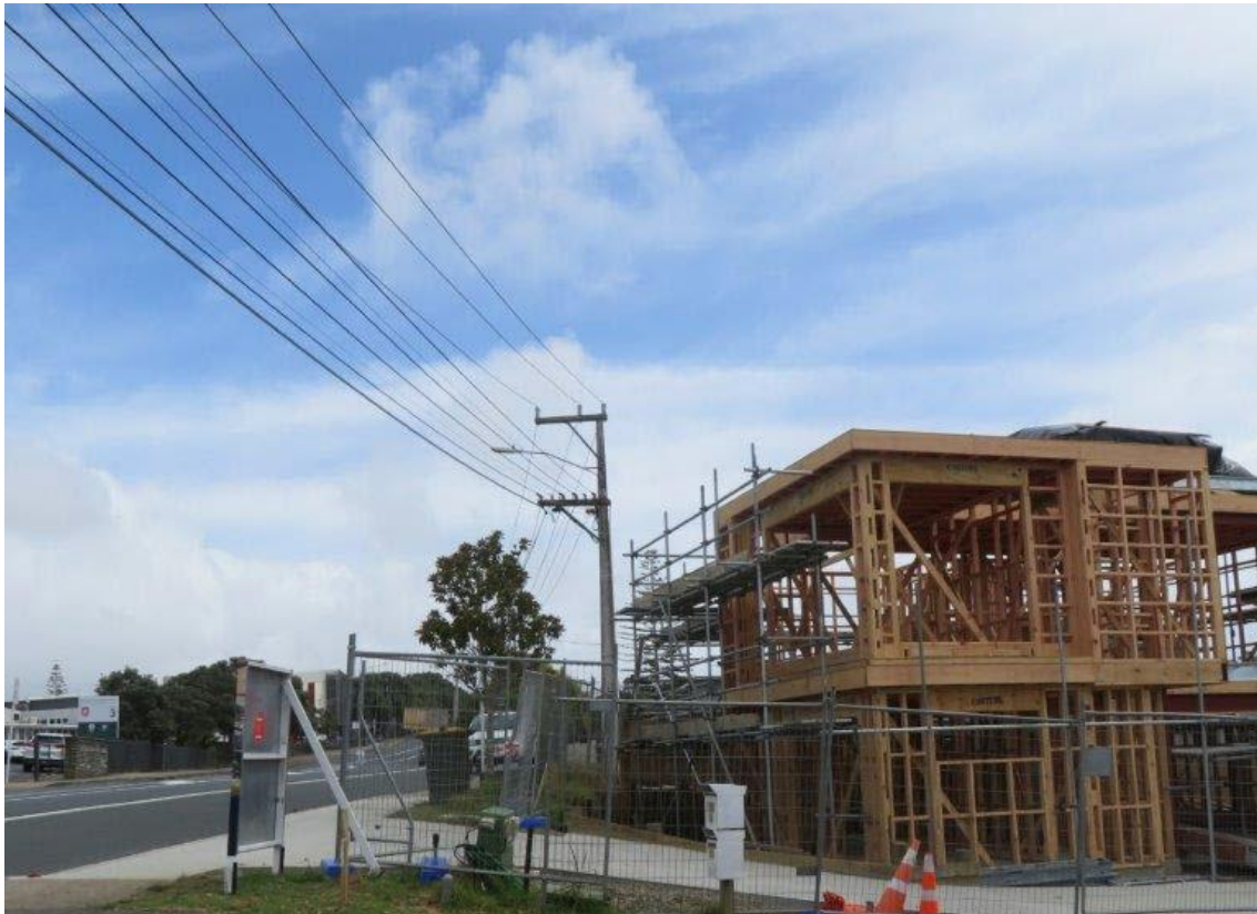
Figure 1: Non-compliant building and scaffold near 400V and 11kV lines – the building had to be partially demolished and re-consented to compliance.
